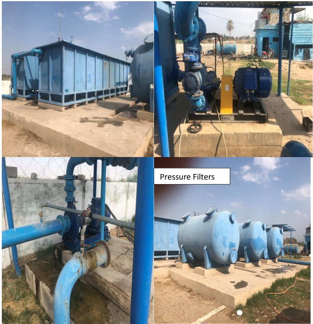
Figure 3: Damage to the Facilities
