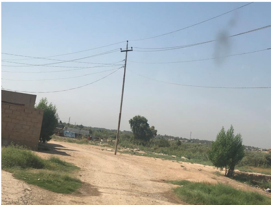
Figure 3: Current situation of electricity grid in Al Ahbab Village
