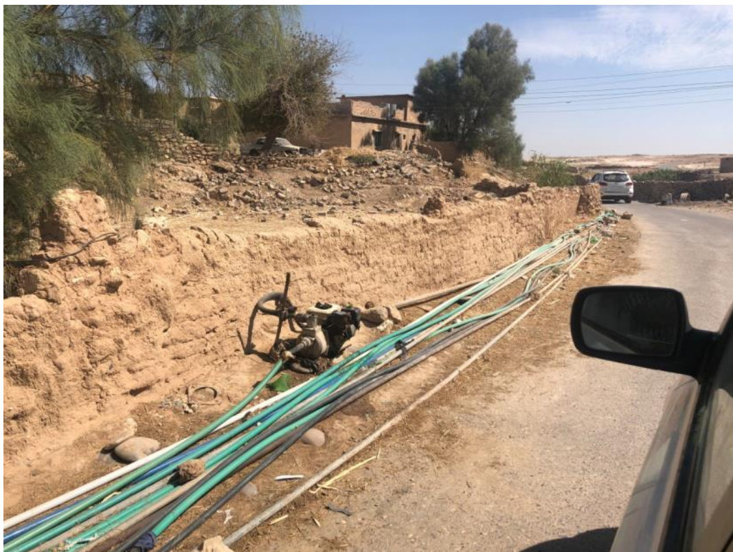
Photo of the current water distribution network
