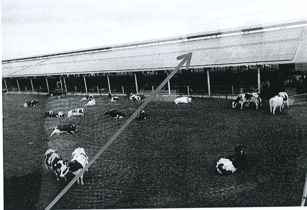
Photovoltaic power generation
