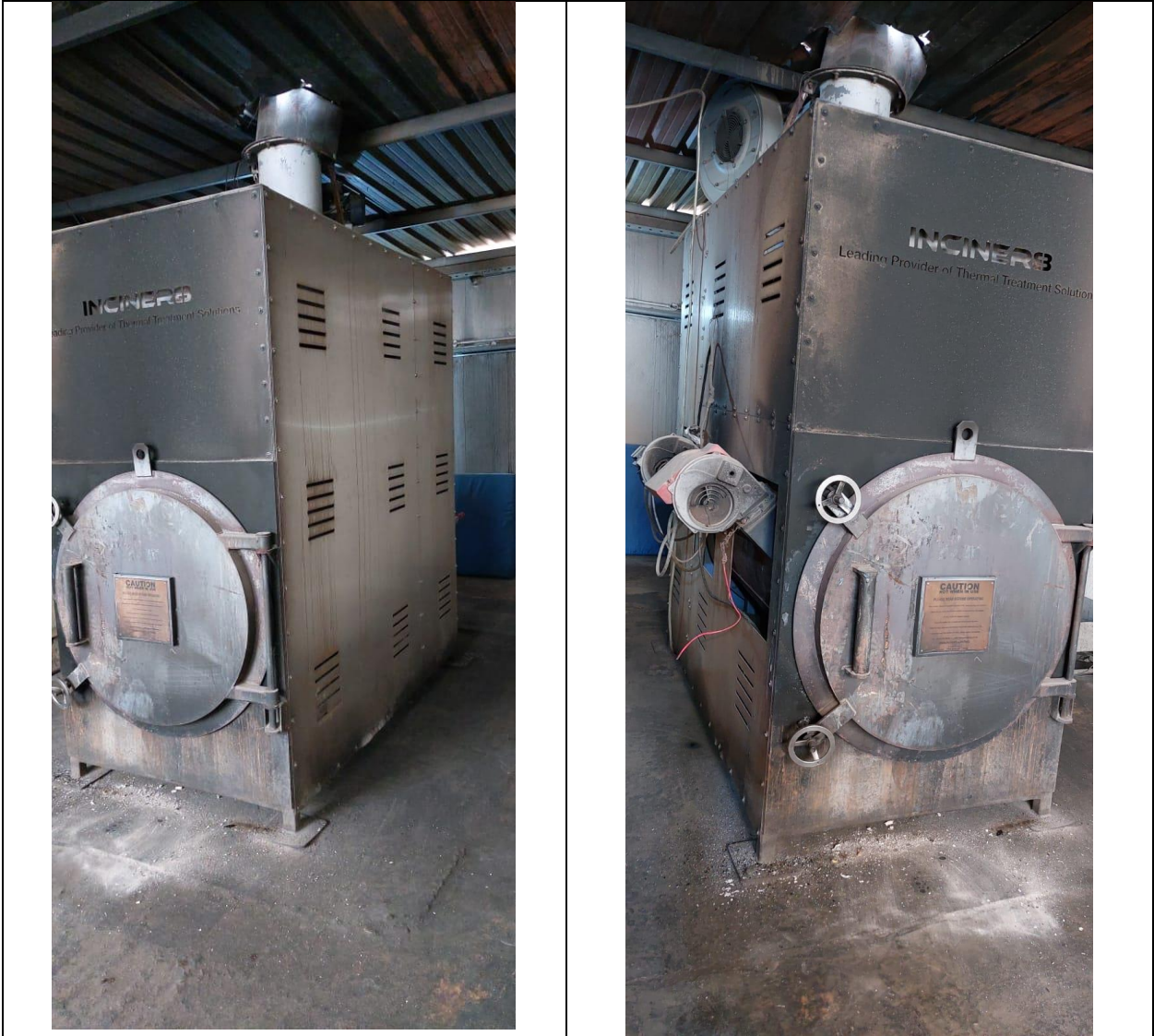
Medical Waste Treatment System
